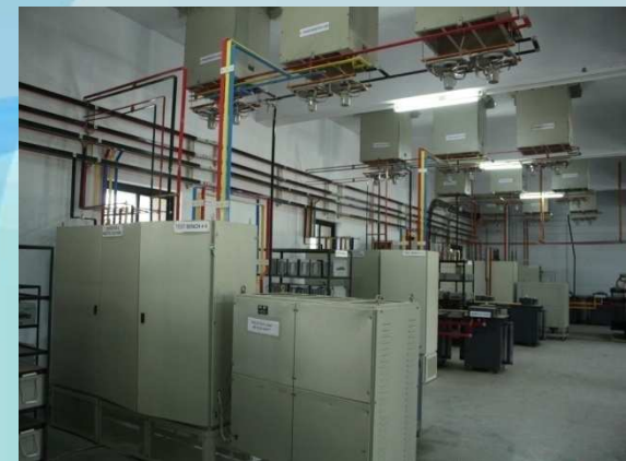
Overview of Load Banks
