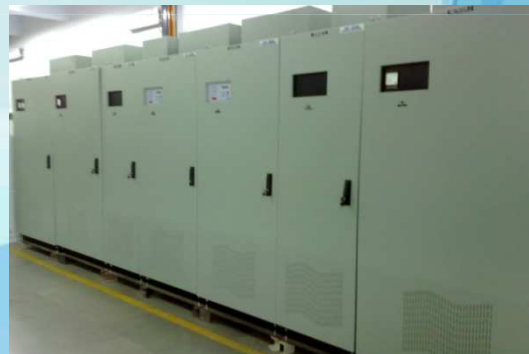
160 KVA System under Testing
