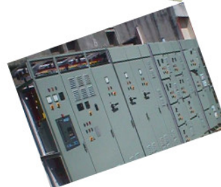
Automation Control Panel
