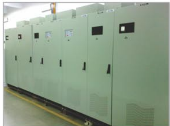
350kVA System Under Testing
